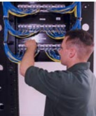
Patch panel termination
